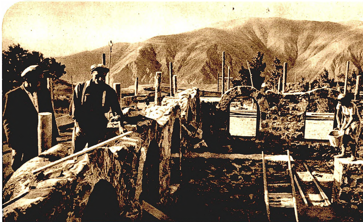
Foundations of a new club in the village of Nor-Avan, Sisiyan District.
