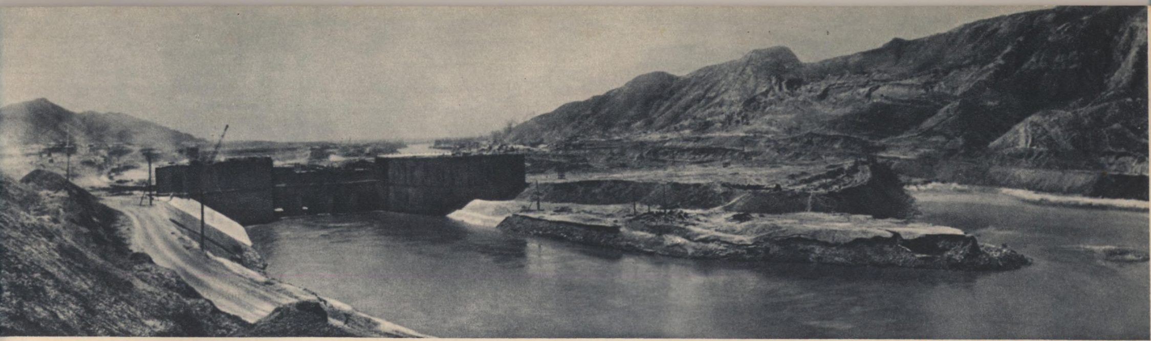
The waters of the Kura do not interfere with the work: In the construction area the river has been dammed up and diverted into ferroconcrete pipes
