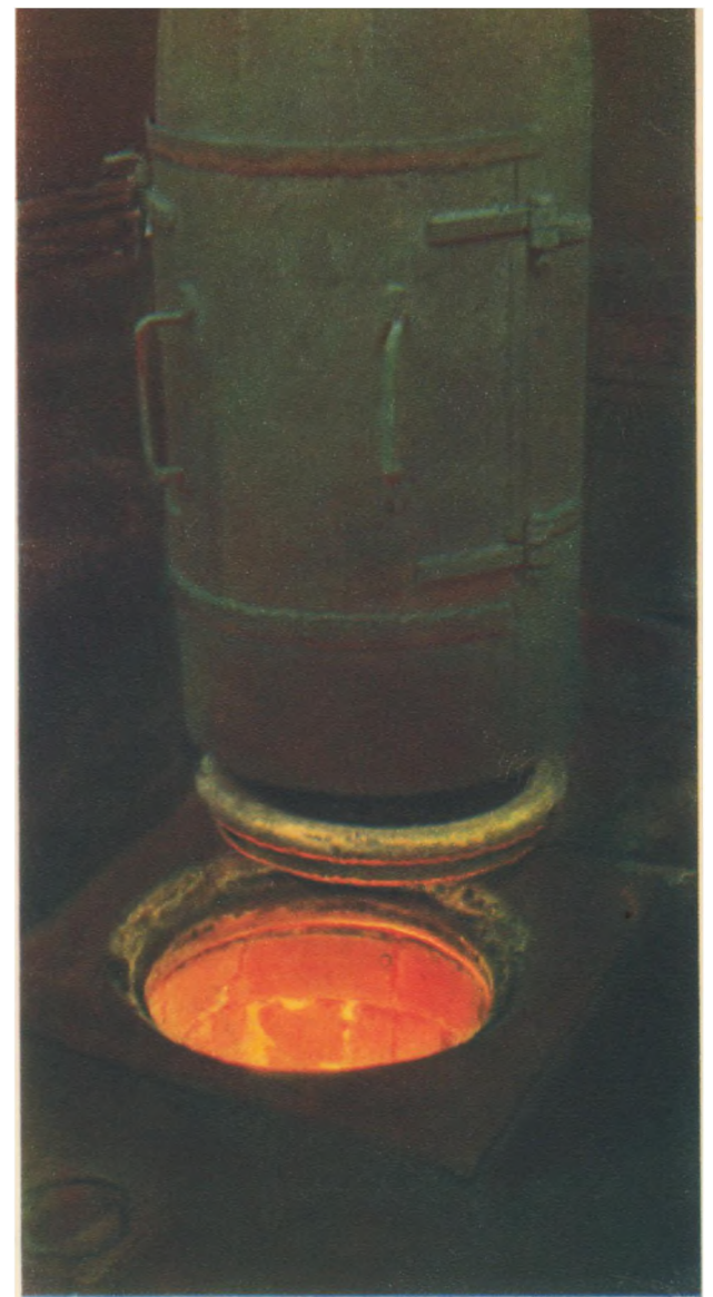
The charging cars at the Zaporozhye Coking Plant are equipped with electromagnets like the one shown above, photographed just as the coke-oven hatch opened
