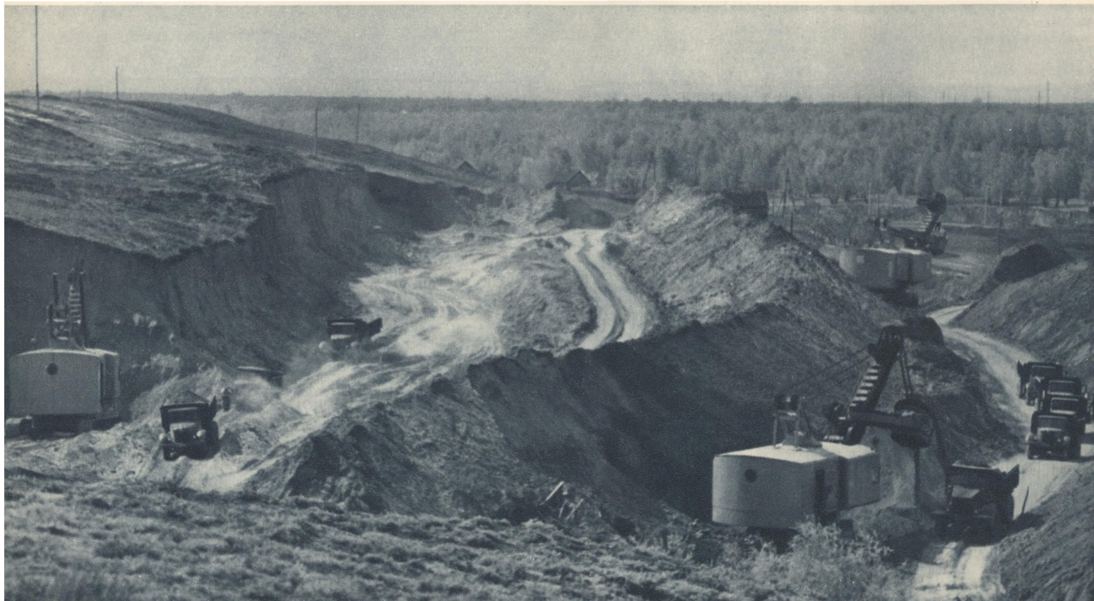
Electrically-powered excavators throw up an embankment round the foundation of the future Stalingrad Hydroelectric Station. On the right, Victor Borisov's excavator works by the highly efficient semicircular method of digging
