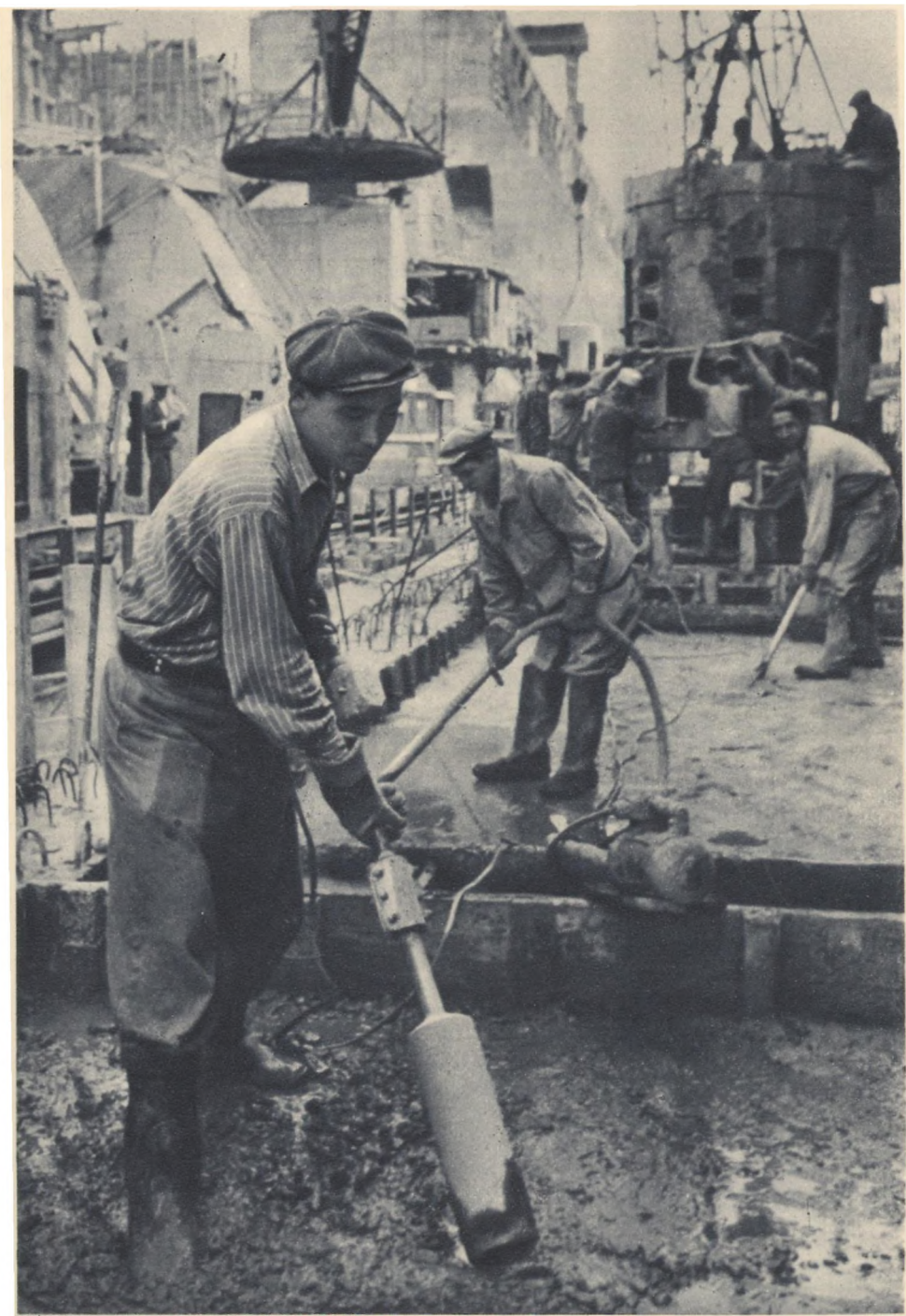
Alibek Altibaev (foreground) and his team lay concrete with the help of electric vibrators
