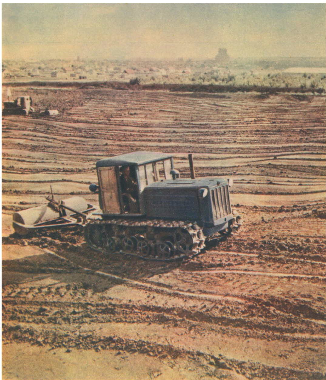
Construction of a pond on one of the 12 collective farms where the Millerovo MTS has helped to dig ponds and reservoirs in the past three years
