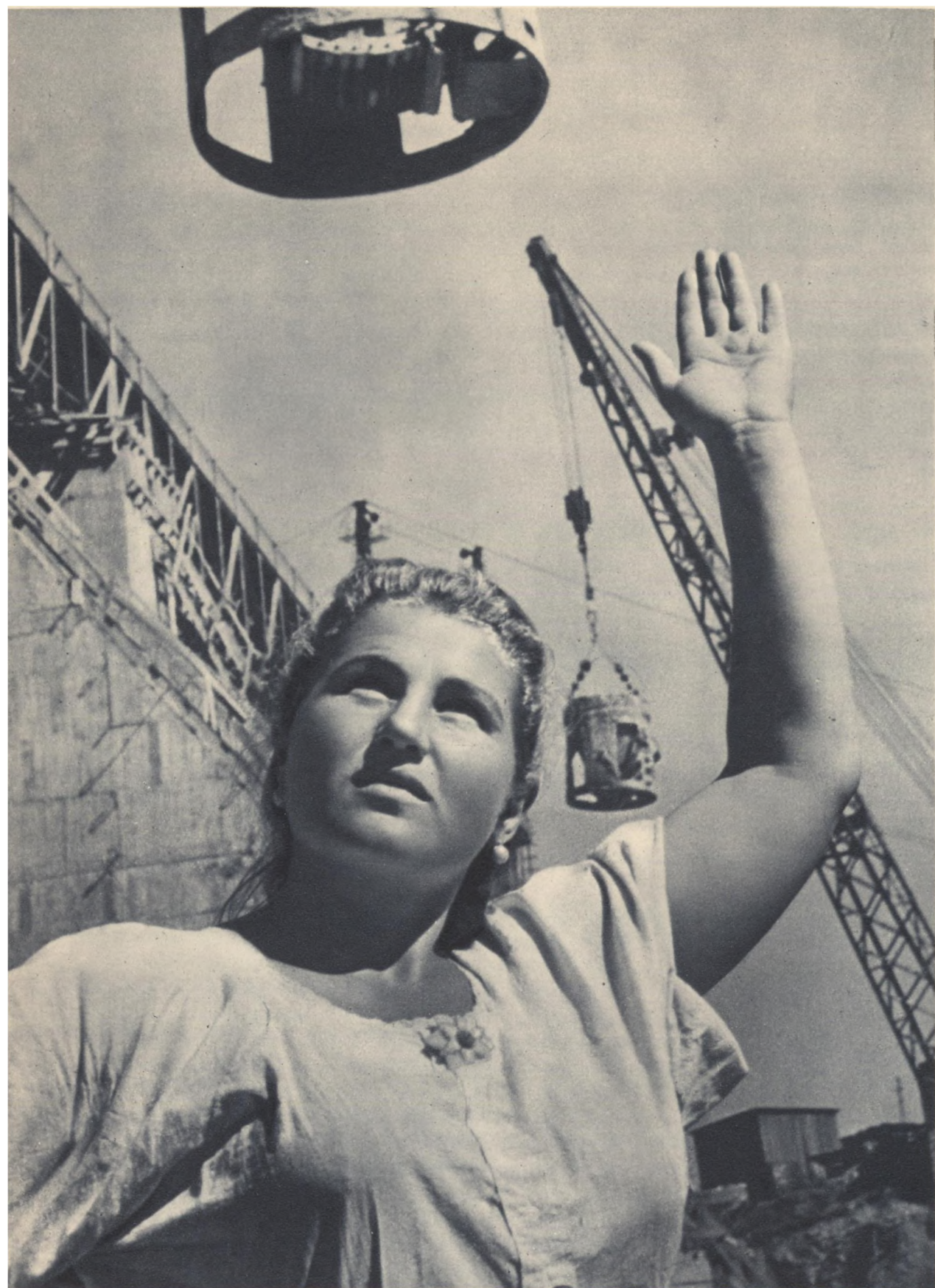
Yekaterina Denisova does a fine job as signalwoman for a concrete-pouring crane
