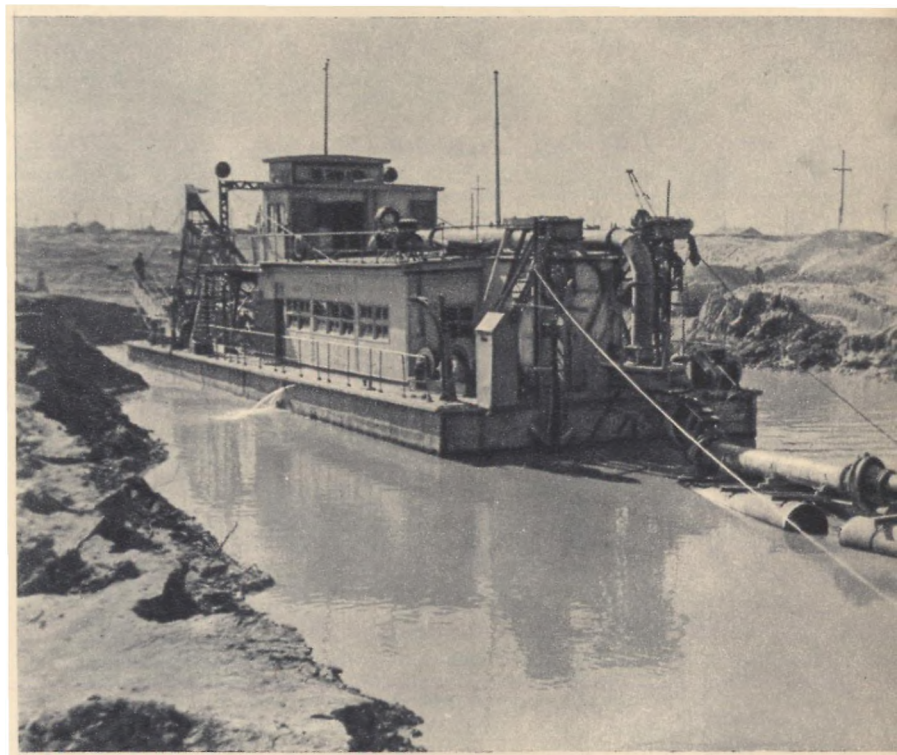
An electric dredger is seen here at work on the construction of new hydropower developments
