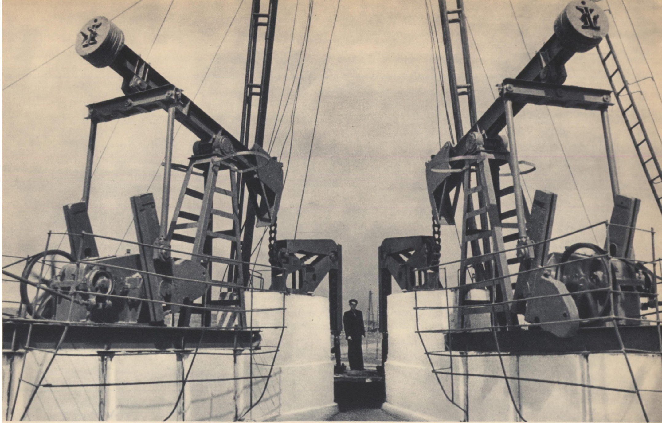
This is the surface machinery of a multiple well; oil is extracted from several strata at a time
