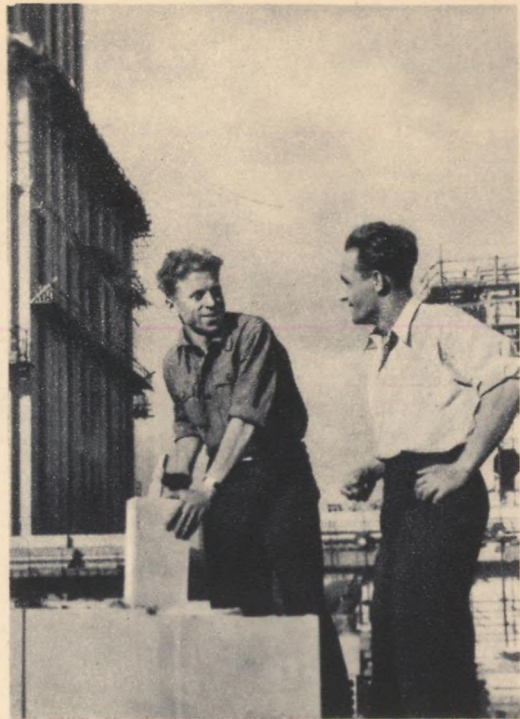
S. Piskun (left) and Nikolai Batsura are building workers at the multi-storeyed hotel going up on Dorogomilovo Embankment in the Soviet capital. Recently Batsura was given the title of Moscow's best facer. Piskun has perfected Batsura's new work methods and achieved a result nearly twice as high: the quota of 19 days in one shift Photo by V. Ruikovich
