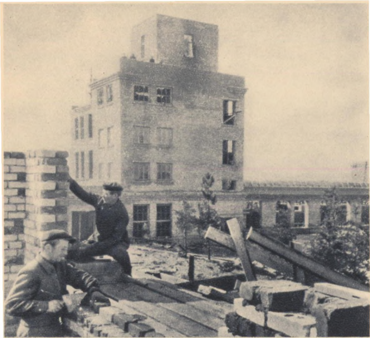
A big factory for making peat insulation panels is being built at Baloži
