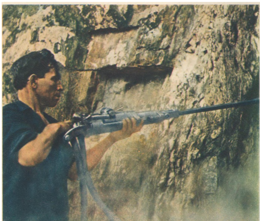
Cutting an adit into the cliff face to enable the geologists to get additional data on conditions at the building site
