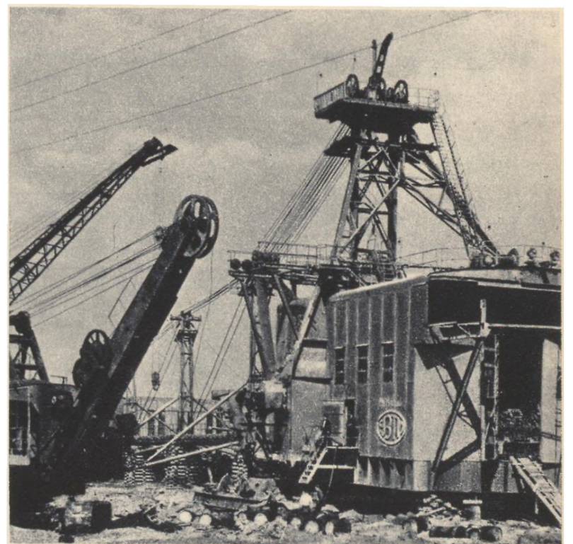
Soviet factories produce new technical aids for the mines of the Vakhrushev field. Here we see a 14 cubic metre walking excavator, brought to the field, in process of assembly
