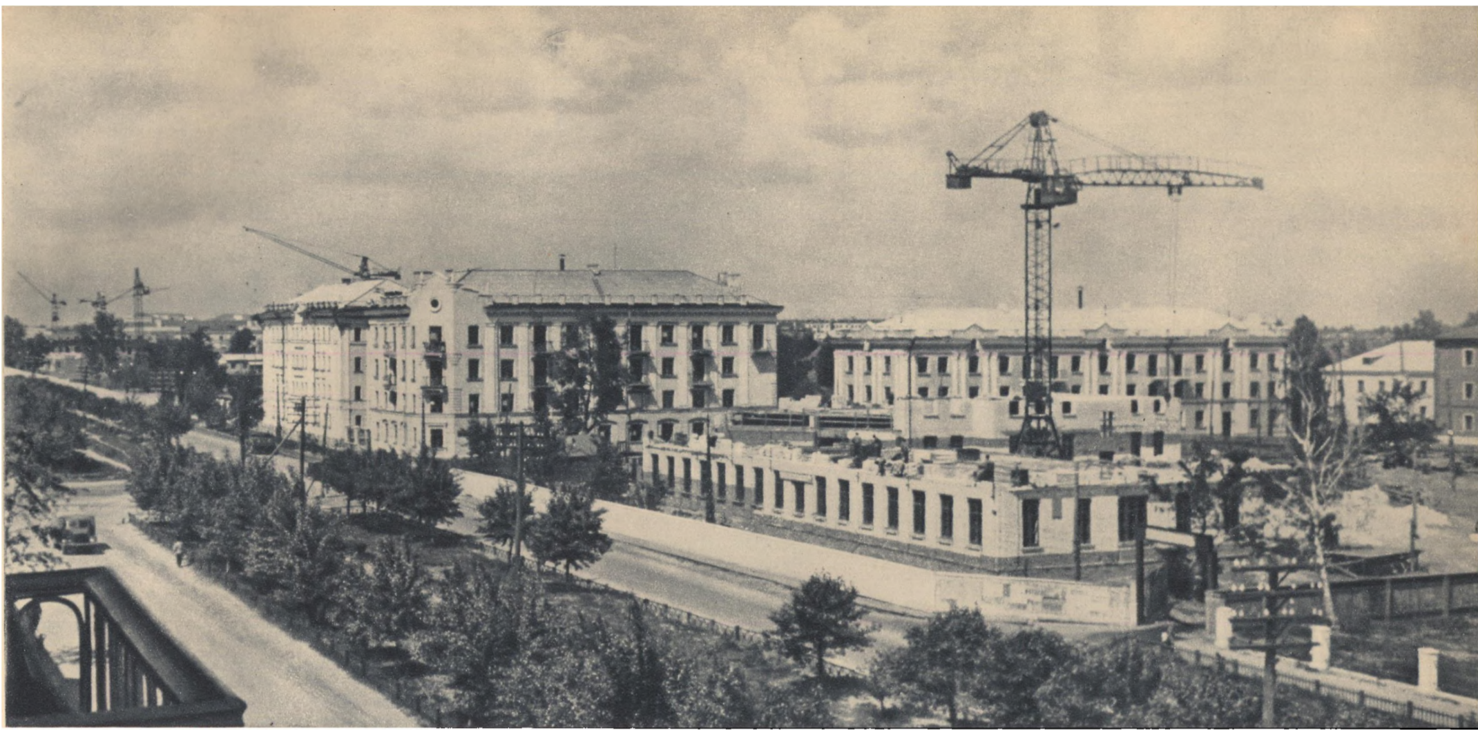
The construction site of a new technical school on Lenin Avenue, one of Barnaul's main thoroughfares, where many new houses are being built
