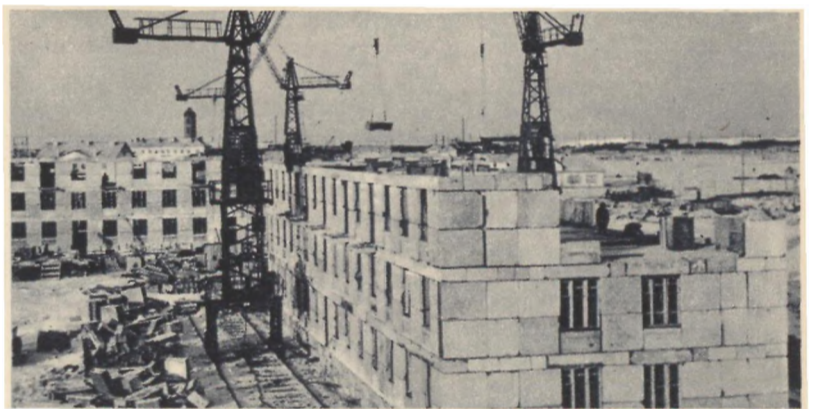
KAZAKH REPUBLIC. This housing estate in Pavlodar is being put up for the workers of the country's largest harvester combine factory, now under construction. The builders of the estate have pledged to exceed the programme in honour of the 20th Party Congress
