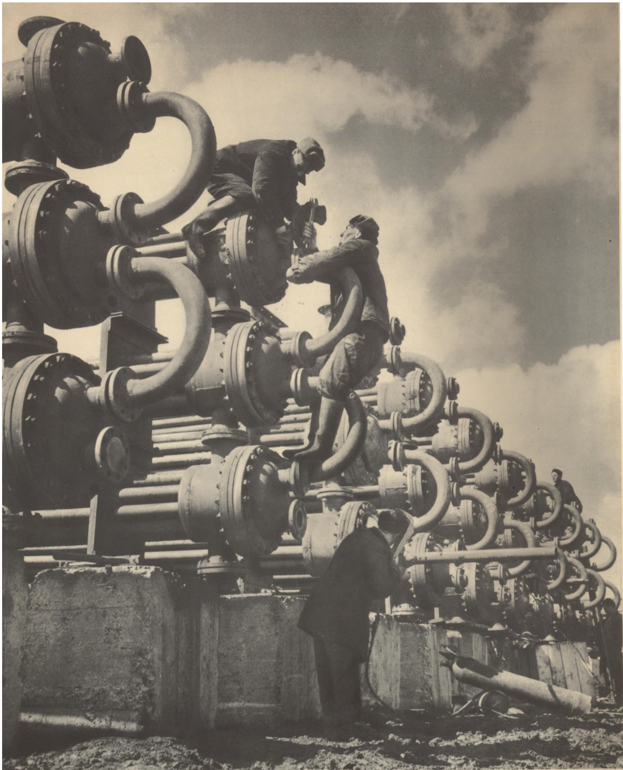
Assembling heat-exchangers at the natural gas drying department along the new Stavropol-Moscow gas pipeline
