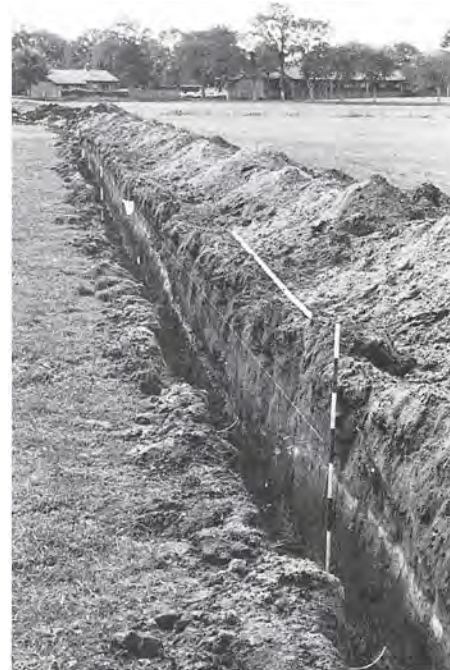
1561:6. Løgumkloster. Trench for natural gas pipe at Sølstedgårds meadow. The bottom deposit in the pit of the rear sluice of the moat system is visible as a greyish layer. Seen from the NW. NTS phot. 1986.
